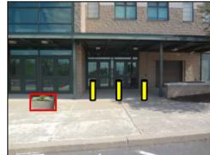
Photo 2: Bollards could be combined with large planters at entrance #5 to prevent vehicle impacts with the school building.
